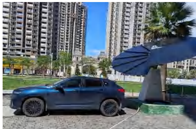
Electric vehicle charging pile
