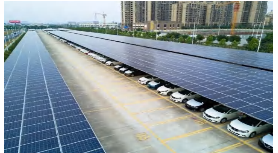
solar parking shed
