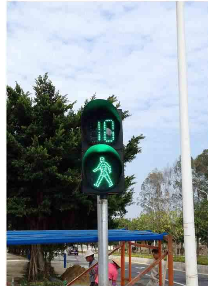
LED Traffic Signal Light in China
