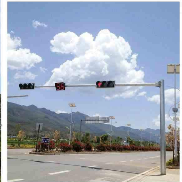
LED Traffic Signal Light in China
